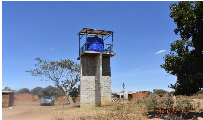
A gravity-fed water pumping system installed at Chimphanga Village
