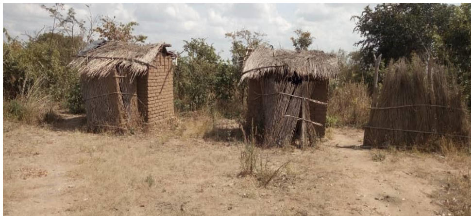
Dilapidated toilets used by learners at Kanjochi Primary School prior to the project
